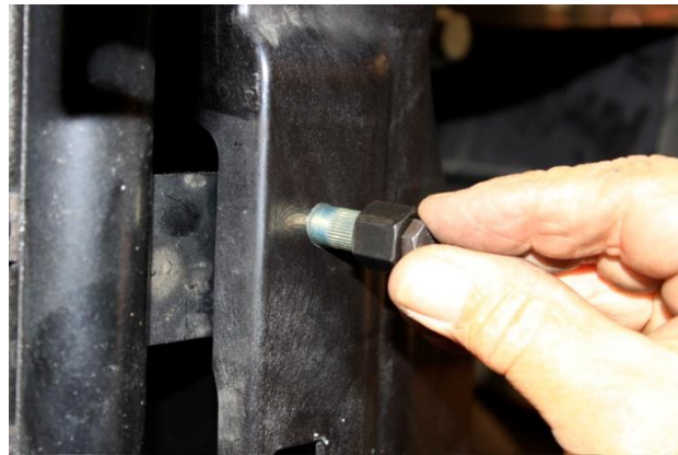
18. Remove mounts and drill hole out to 25/64". Install Nutsert using supplied setting tool (see separate tool instructions).
